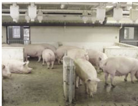
There are many different feeding systems, the drop feeding system being the cheapest way to retrofit a barn
